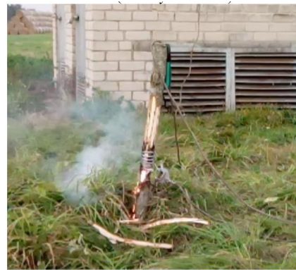
Figure 19 Test site for high impedance fault
