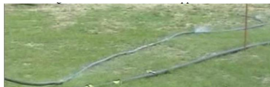
Figure 10 Overhead line touching the ground (gras) – parallel connection of many fault points
